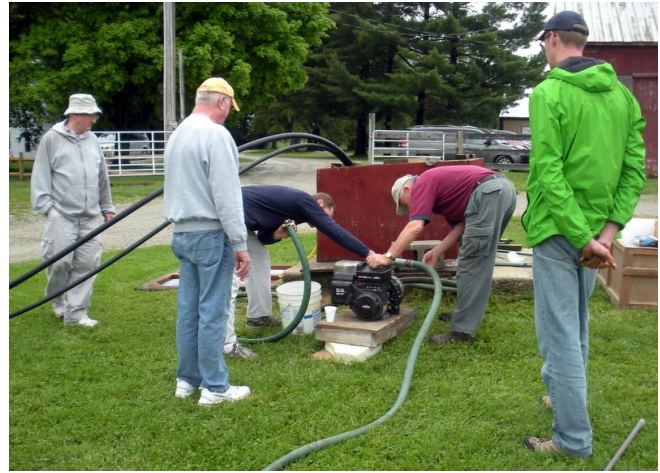
Members of the 3rd Saturday Crew even pumped water out of the well using another pump to get the level low enough to see the pipe through which the suction lines had to pass to reach the bottom of the well. Photo: JCD
