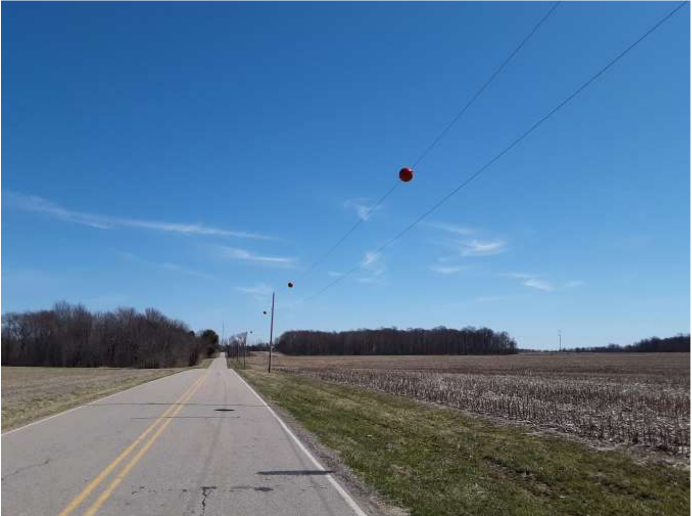
Newly installed electric wire safety balls along Gard Road, south-east corner of field.
